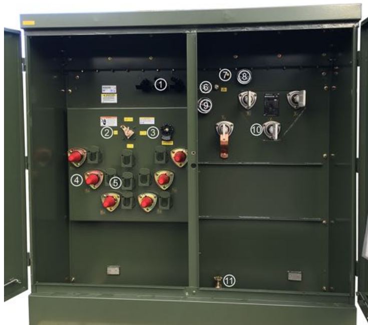
Fig 2. Three Phase Maddox Padmount Transformer
